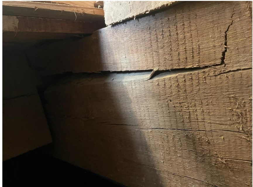
View the cracked fireplace header, which supports three levels of brick masonry.
