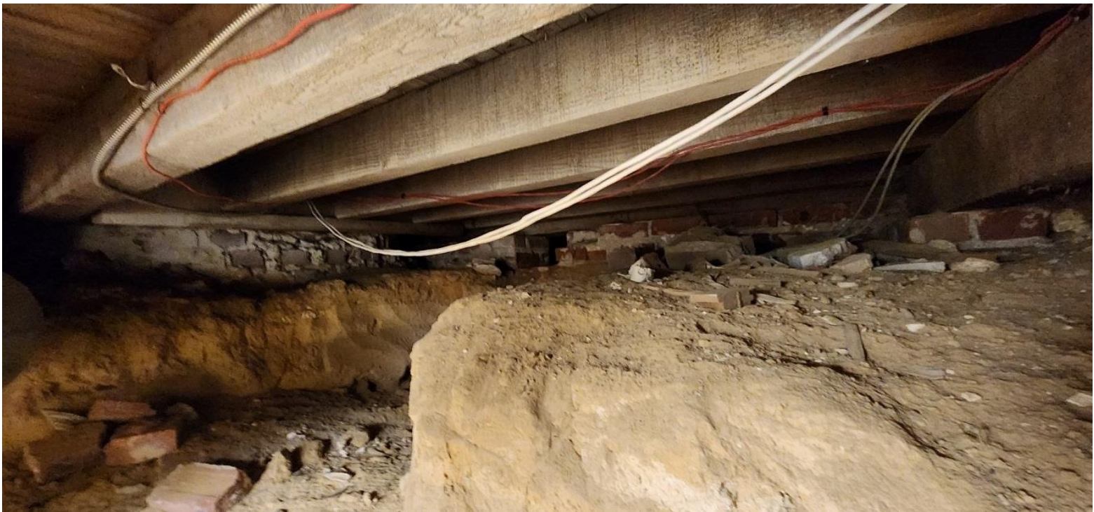
View of the crawlspace looking northeast showing how portions of the crawlspace have been dug out.
